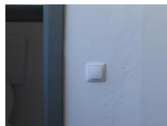
FIG. 21 - Interruptor na IS
